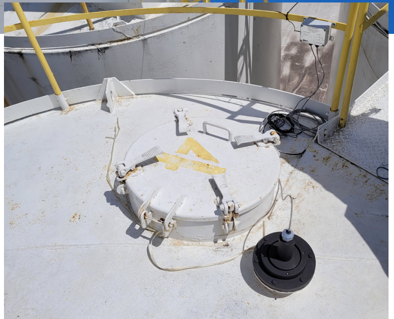
Figure 1: ABM's Ultrasonic Level Sensor and Cellular Gateway installed on top of the tank.
